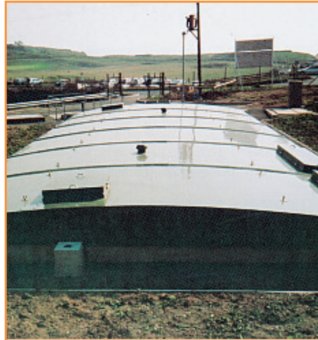
■ Six Section Cover for a storm storage tank
